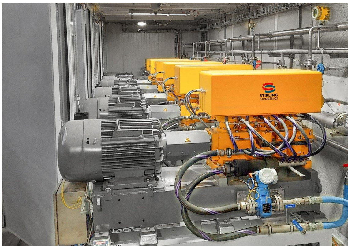
Containerized liquefaction system
