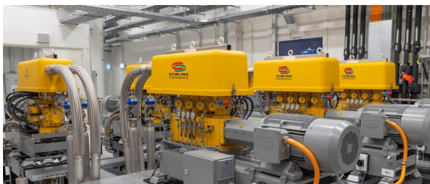
2019 Stirling Cryogenics Hydrogen Re-liquefier for Cold Neutron Source at RID Photo Courtesy Reactor Institute Delft, The Netherlands
